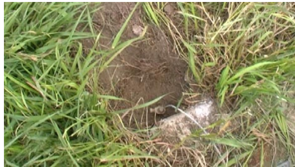
Figure 8. Machine ground of Reinke unit to ground stake.
