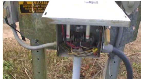
Figure 3. Power supply to Valley Pivot. Valley Pivot plugged into receptacle.
