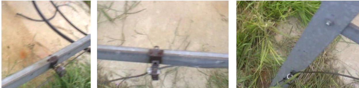
Figures 5-7. Path of Reinke ground wire.
